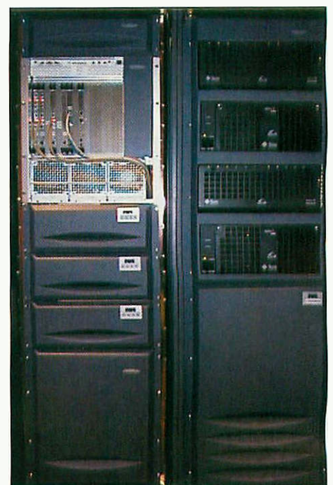
Cisco routers like these are being installed at BT Cellnet radio sites across the country.
