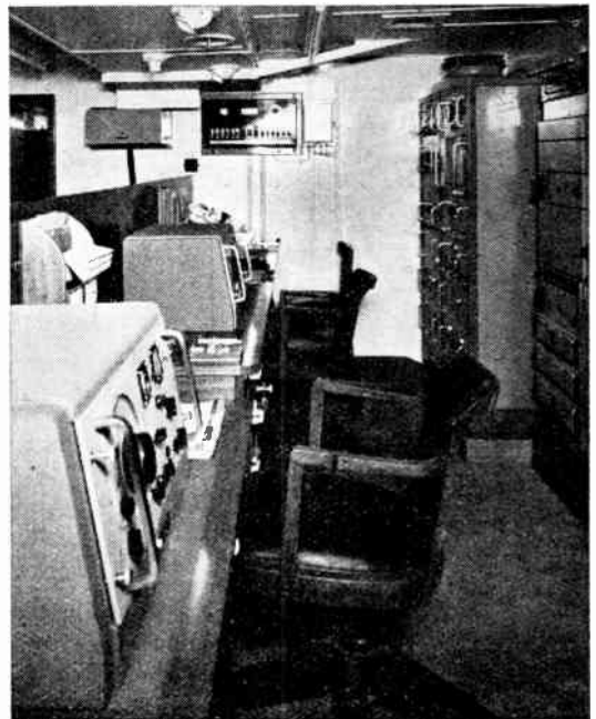
Two of the receiving positions in the Caronia . The single sideband receiver is seen in the right rear alongside the telephone terminal equipment
