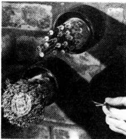
This optical cable being held has a bandwidth greater than the 4800 pair cable or the 18-core 9mm coaxial cable. The space requirement is tiny compared with the other two types of cable.
