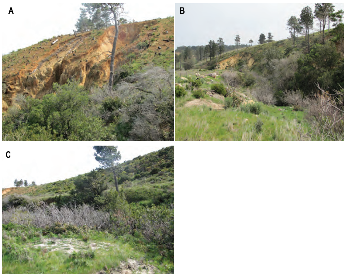
Figure 3.6: Sir Lowry's Pass River site (cleared). (A) river bank erosion; (B) riparian zones supporting high grass cover and (C) scars present in terrestrial zones caused by slash that was burned in piles.
