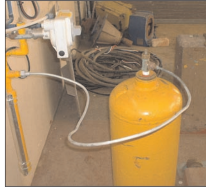
68 kg CHLORINE CYLINDERS
