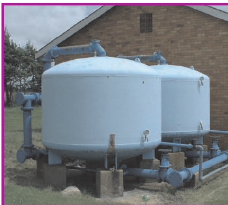
VERTICAL FILTRATION TANK
