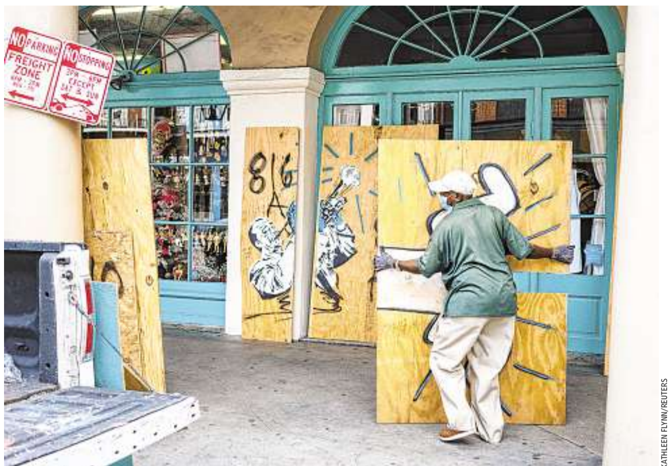
City of New Orleans worker Louis Marrero boarded up businesses in the French Quarter on Monday.
