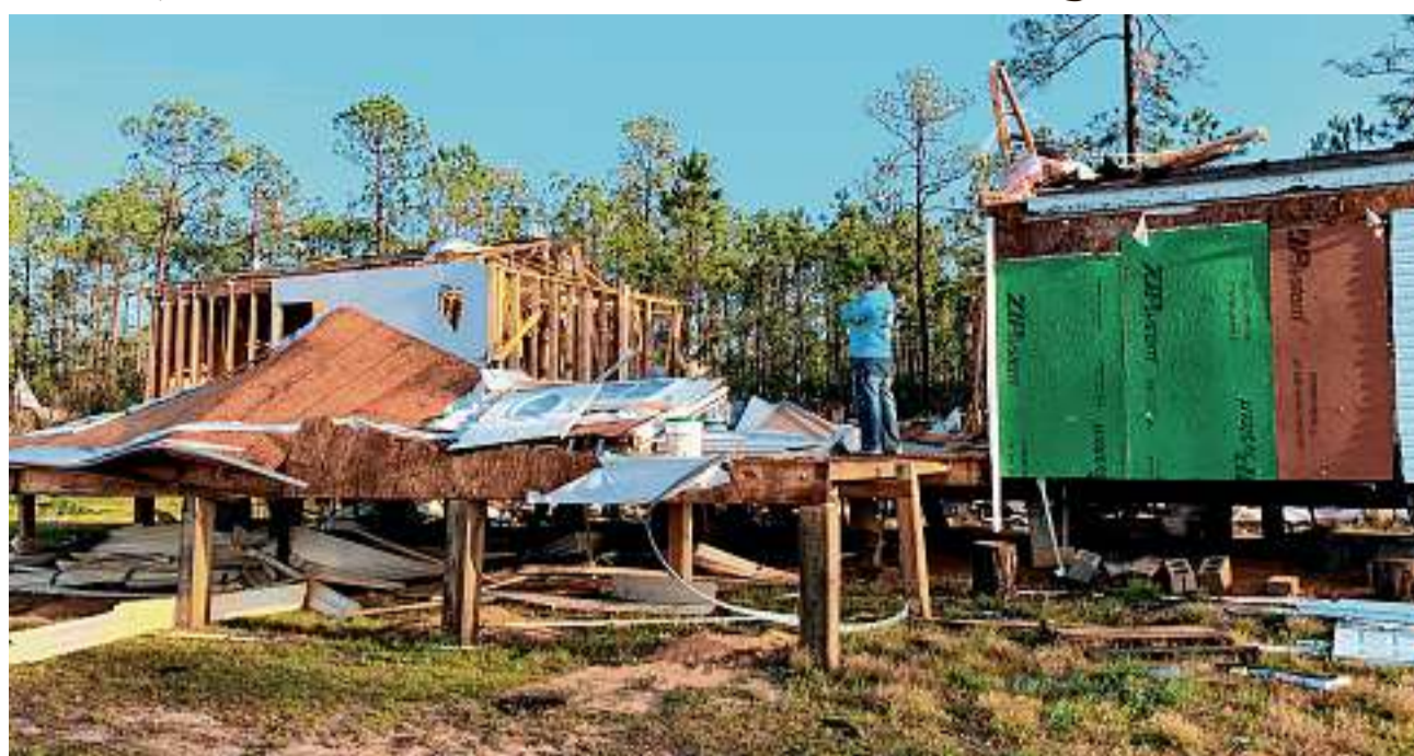
DEMOLISHED: Homes in Vanclave, Miss., were blasted by a tornado, one of at least two in Mississippi and Tennessee on Wednesday. In the western Florida Panhandle, a twister killed two people, while thousands were without electricity Thursday in several states.
