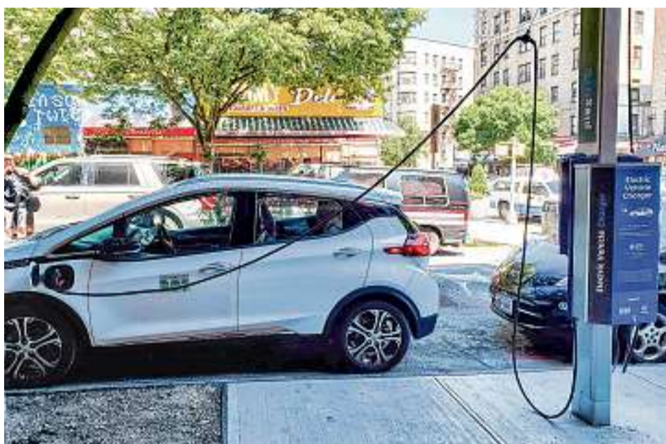
The first of the city's electric-vehicle charging stations was installed in the Bronx's Norwood section.
