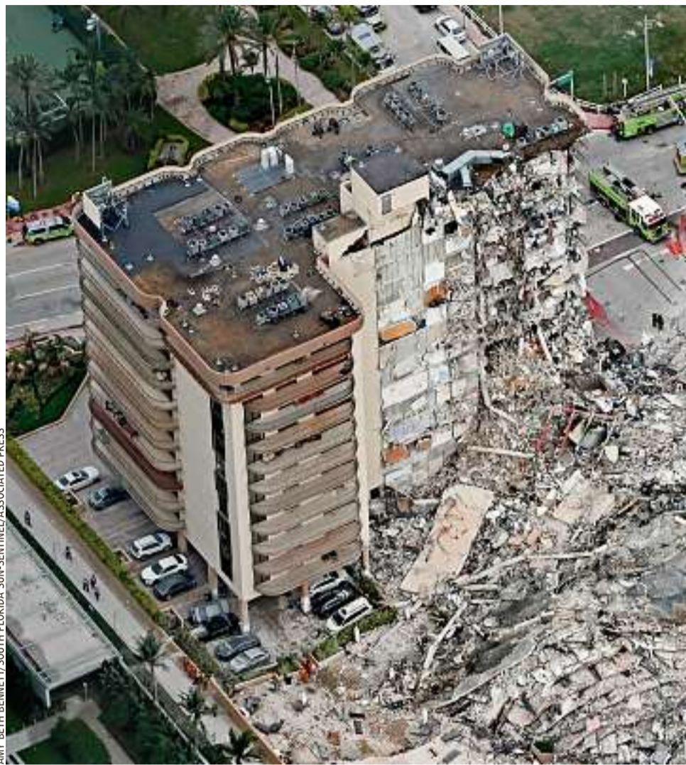
At least 99 people were unaccounted for and one was dead Thursday after a 12-story section of Champlain Towers South in Surfside, Fla., crumbled. Rescuers in the Miami-area town were sifting through the rubble of the 40-year-old building for signs of life.
