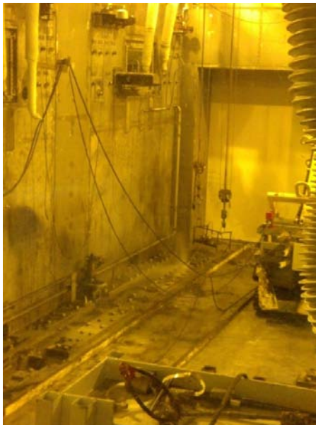
VIT Cell after Clean-up
