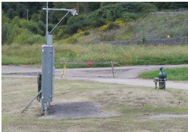
Well 1 and Electrical Panel for New Drinking Water Supply
