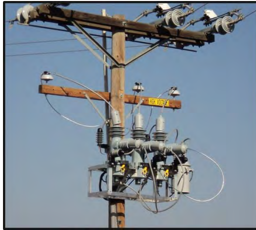
Recloser on Distribution Pole
