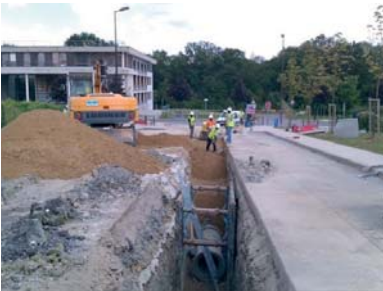
Drainage works at Cluster Descartes in Marne la Vallée (77) - Ateliers Lion Architects
