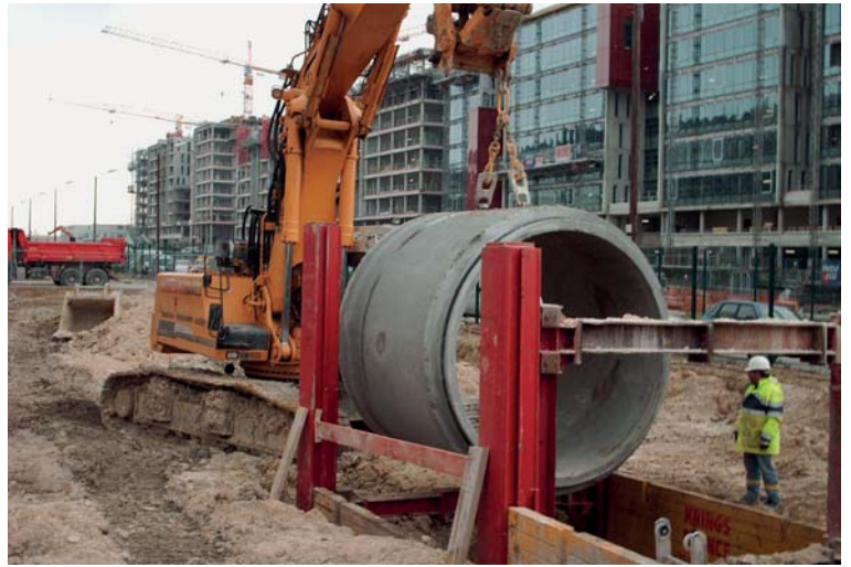
Drainage networks at Seine Arche District in Nanterre (92) TGT Architects
