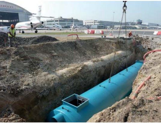
Oils separators setting in restricted areas at Le Bourget Airport (93)
