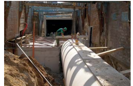
Construction of a pipe gallery and utility network displacement at la Pitié-Salpêtrière Hospital in Paris (75)
