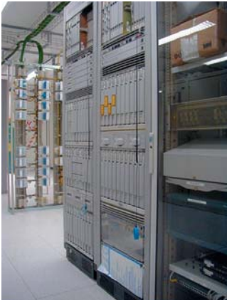
19 telecommunications centres in France for Lambdanet, Internet network provider
