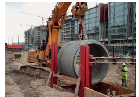
Drainage networks at Seine Arche District in Nanterre (92) TGT Architect
