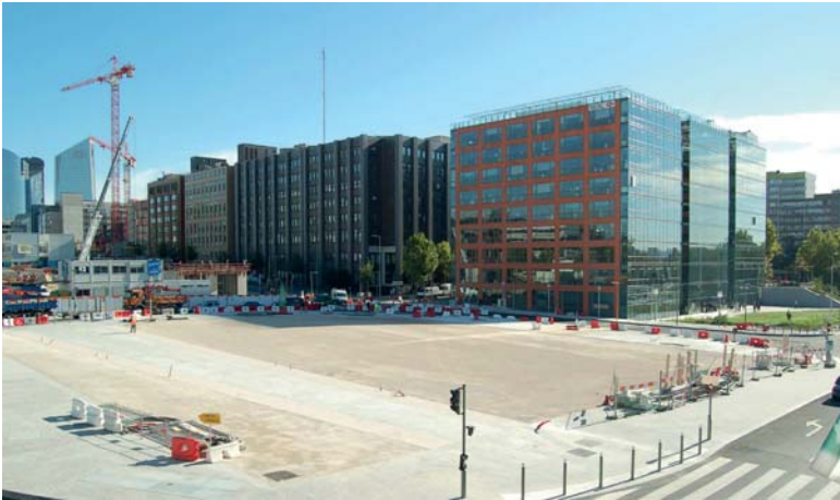
Laying out of a public area of Seine Arche District in Nanterre (92) TGT Architect and Planner
