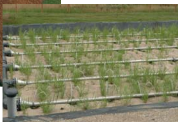
Alternative wastewater treatment process at Bougainville High School in Brie-Comte-Robert (77) Ateliers 234 Architect
