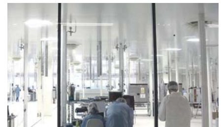
Controlled atmosphere area for EFA Medical SORIN Group in Clamart (92), ABH Architect
