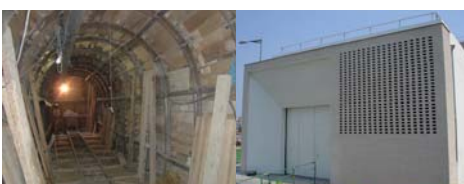
Relocation of electrical of RER Regional Express Network in Nanterre (92) - TGT Architecte
