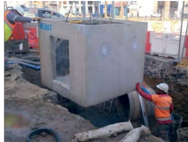
Laying out of du François Mitterrand mail in Rennes (35) - Mutabilis Landscape Architect
