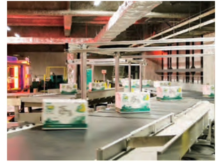
13—Cross belt sorter at Chubu Gateway, with a sliding base mechanism that doubled the previous processing capacity
