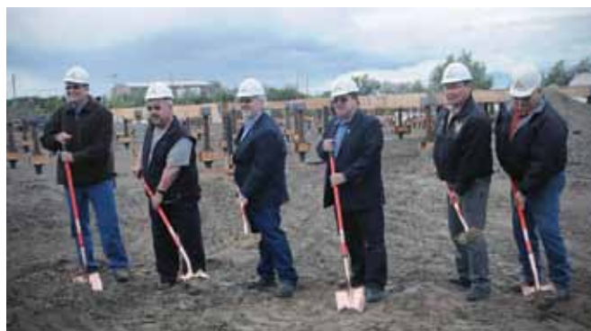
Breaking ground for the new Long Term Care facility. YKHC Vice President for Support Services Greg McIntyre, President/CEO Gene Peltola, Rep. Bob Herron, Senator Lyman Hoffman, YKHC Board Chair Ray Alstrom, Board Vice Chair Bill Kristovich.
