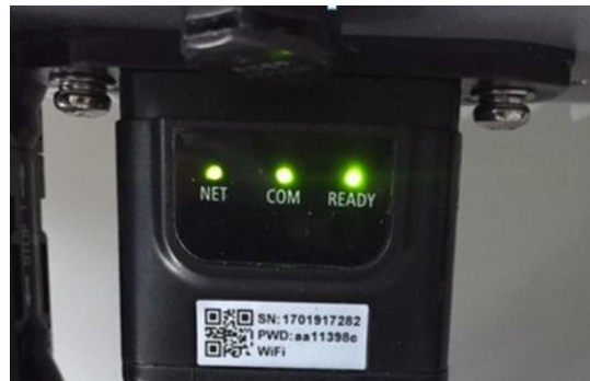
Figure 90 - Final status of LEDs
