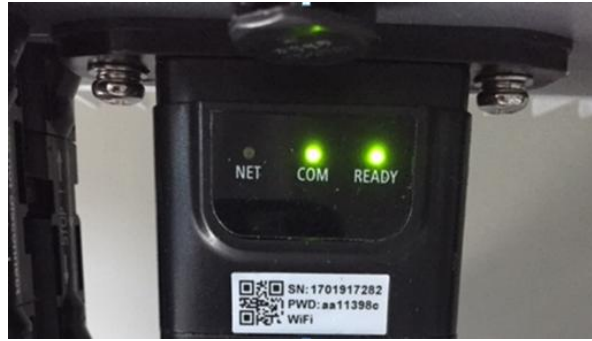
Figure 89 - Initial status of LEDs
