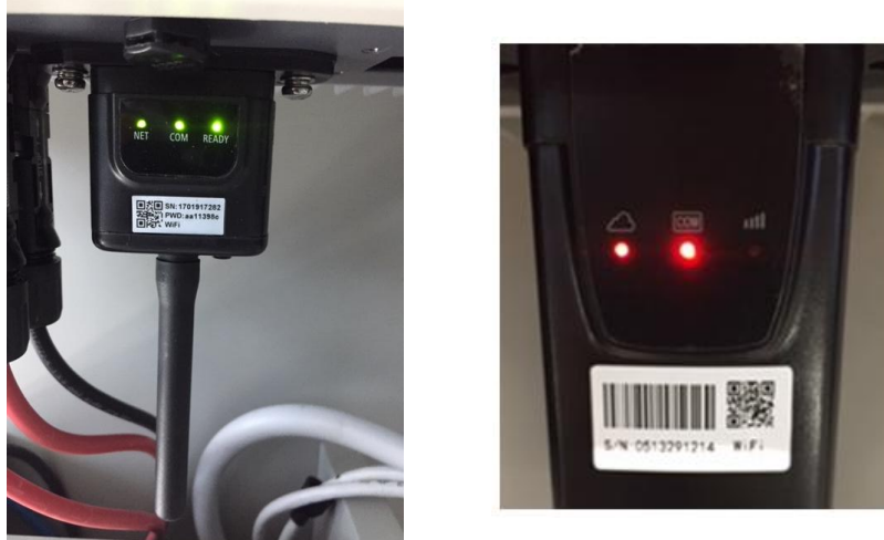
Figure 72 - Final status of LEDs
