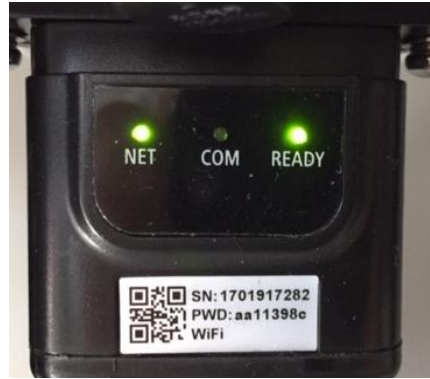
Figure 91 - Irregular communication status between inverter and adapter
