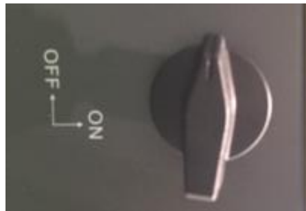
Figure 48 - Photovoltaic disconnecting switch
