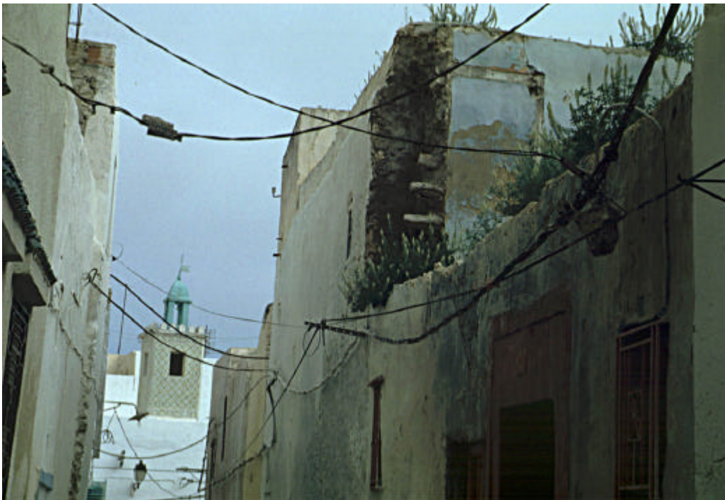
Fig. 4: Wall flora on demolished buildings.
