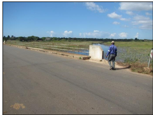
Figure 22: The double lane R241 Inhassoro road as it crosses the Govuro River in 2018
