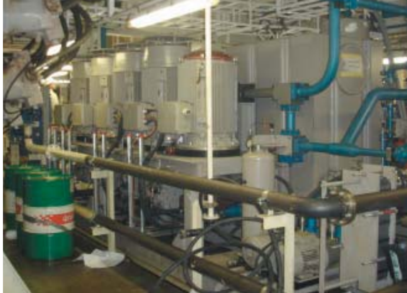
Bosch Rexroth supplied the hydraulic installation
