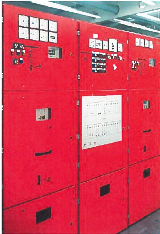
Switchboard: 10 kV High Voltage
