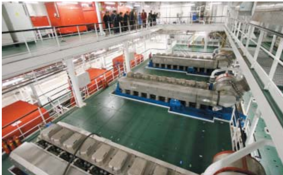
One of the two added engine rooms
