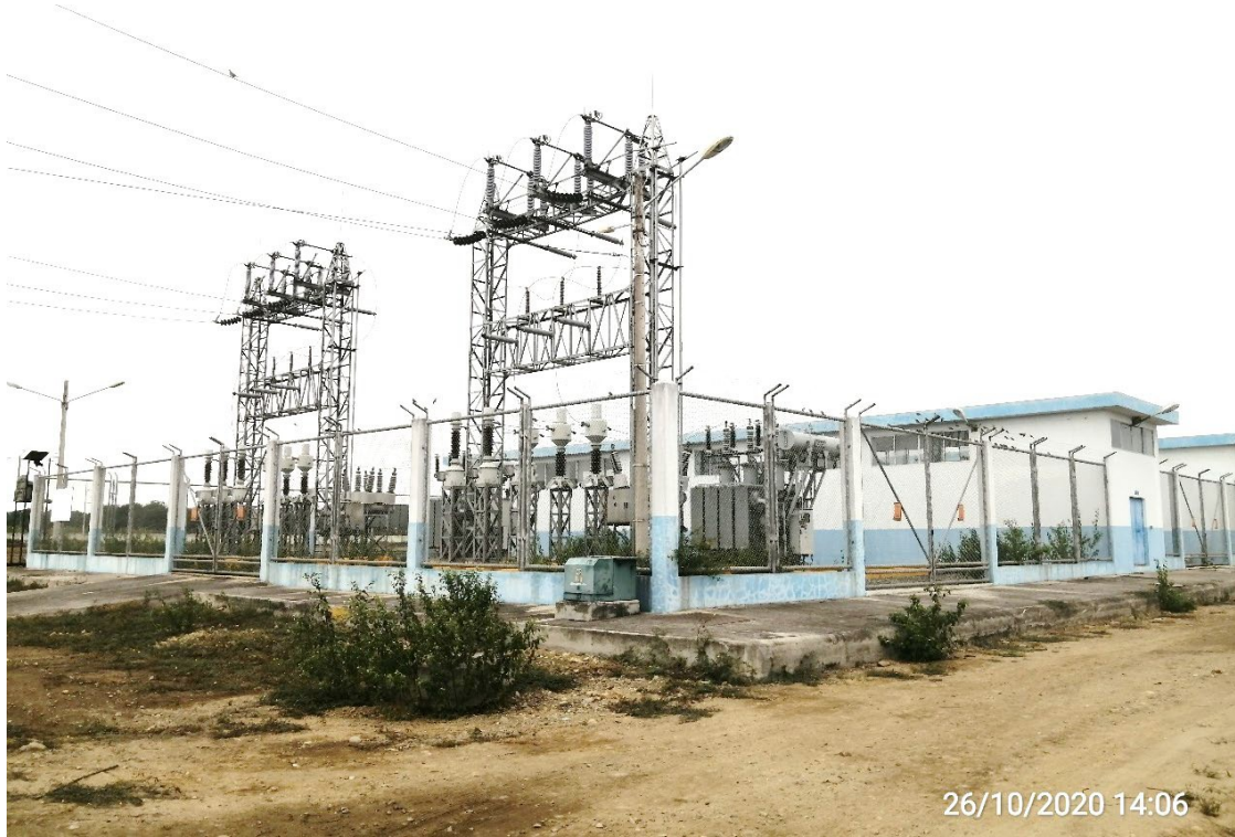
Electrical substation, built in 2012
