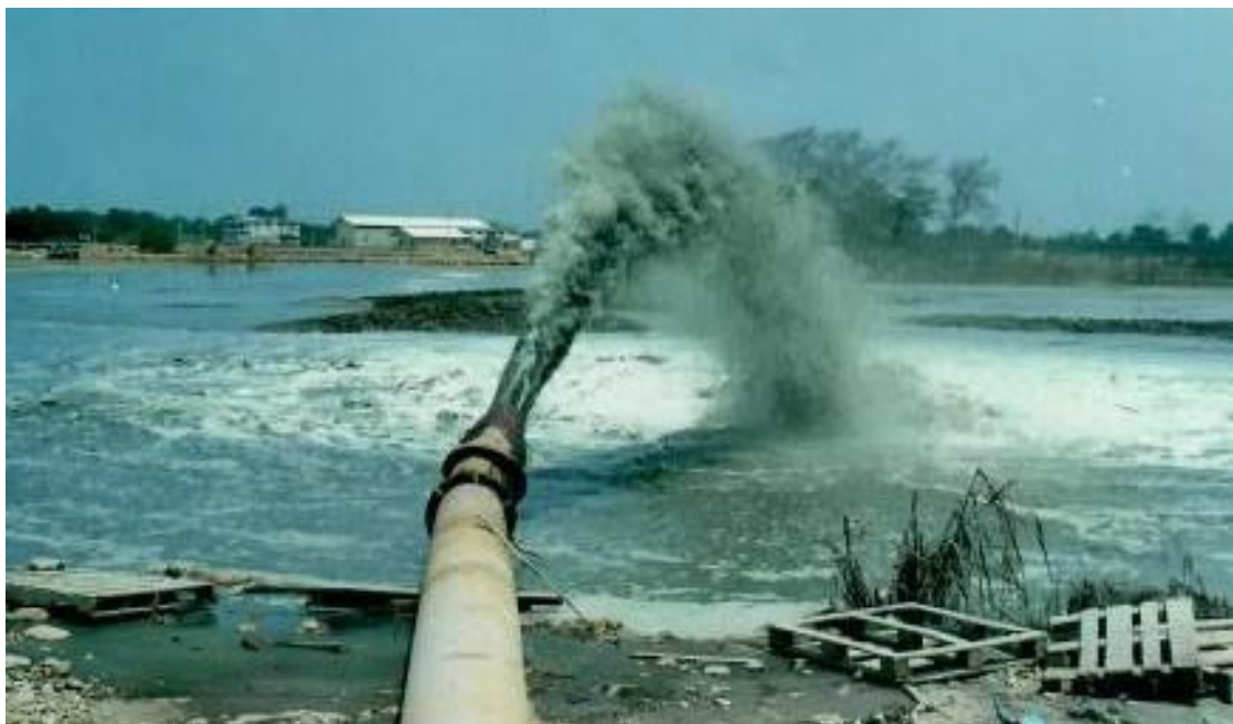
Dumping of sediments dredged from the piers in the sediment ponds, between 2004 and 2009.
