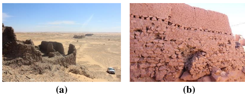
Figure 9. Ighamawen built above rocky hill as foundations: (a) Without earth working in Ksar Aghlad; (b) Built foundations on rocky hill in Agham Basamad Daldoul (photos by Y. Kassou).
