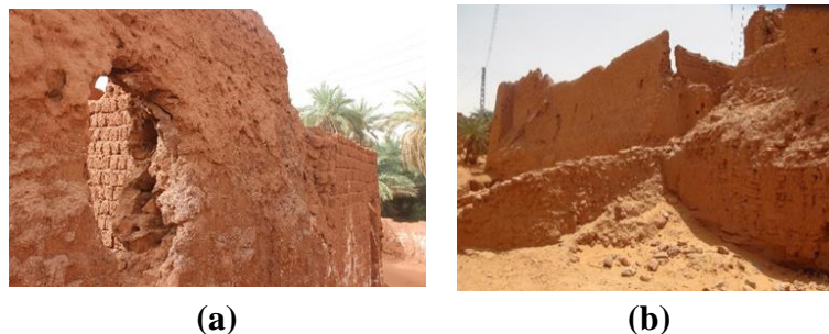
Figure 15. Mixed walls: (a) Mixed walls using salt stone in Agham Sidi Belkacem Ouled Abou Daldoul; (b) Mixed walls using stone, mud bricks in Agham Am'zaghakh Ksar Massine (photos by Y. Kassou).
