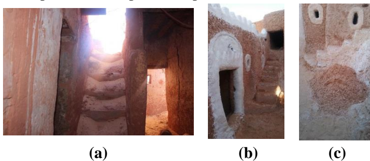
Figure 23. Built staircase: (a) Between two walls; (b), (c) Between wall building and half wall in mosque of Agham Al-Gabli Talmine (photos by Y. Kassou).
