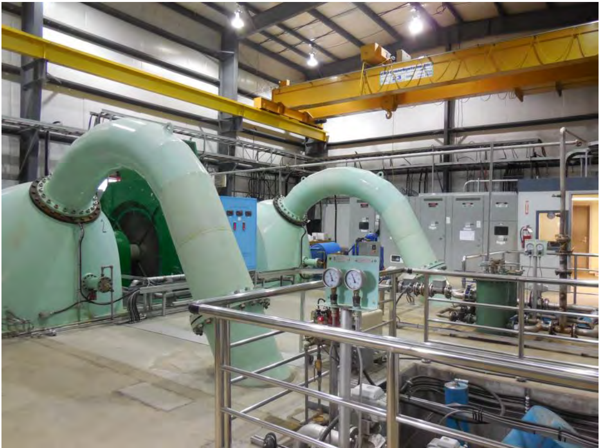
Photo 8: Interior of existing powerhouse showing turbines and crane, looking north. Control room is to the right.
