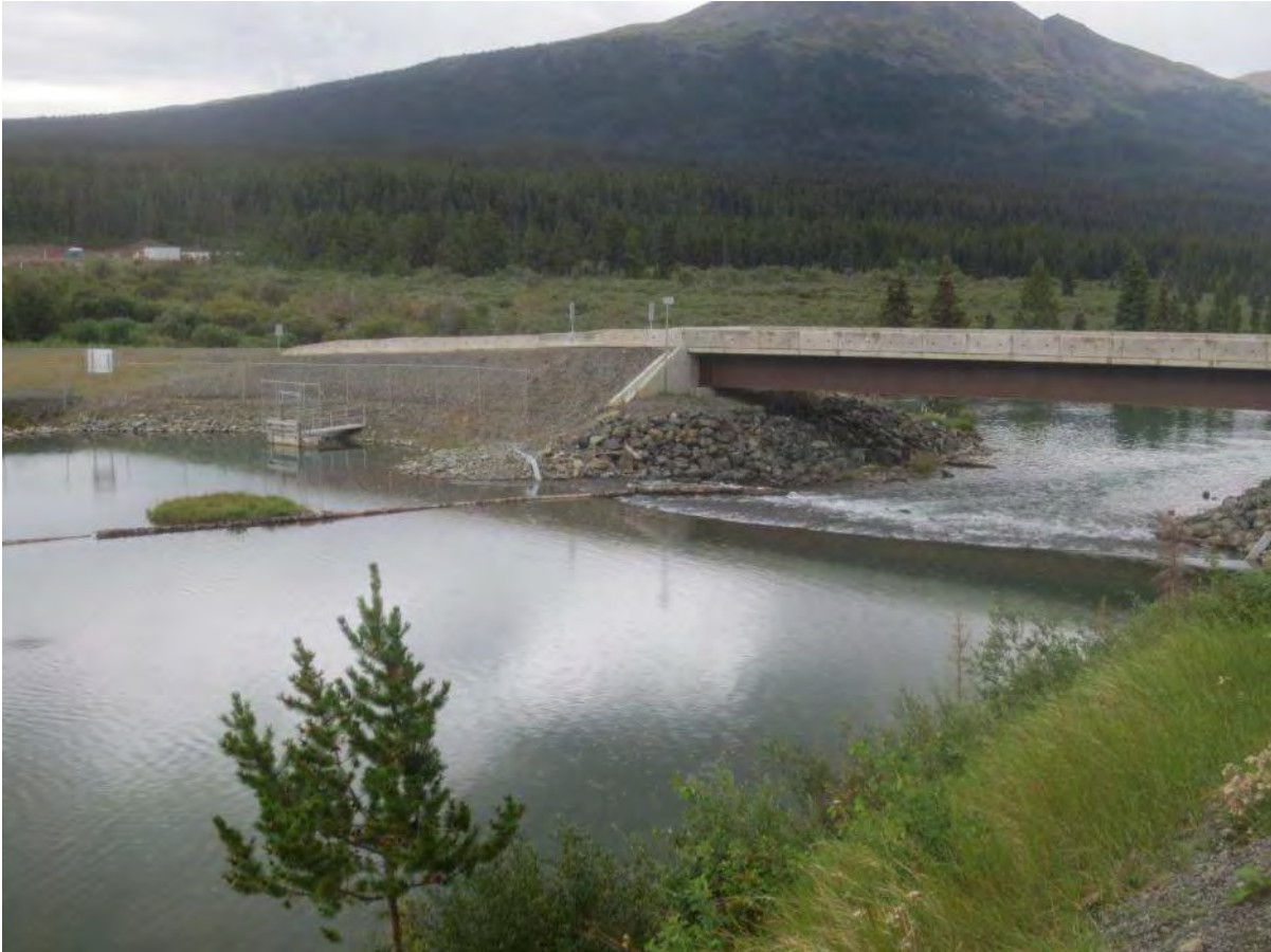
Photo 1: Surprise Lake control structure with rock fill and sheet pile weir on the right.
