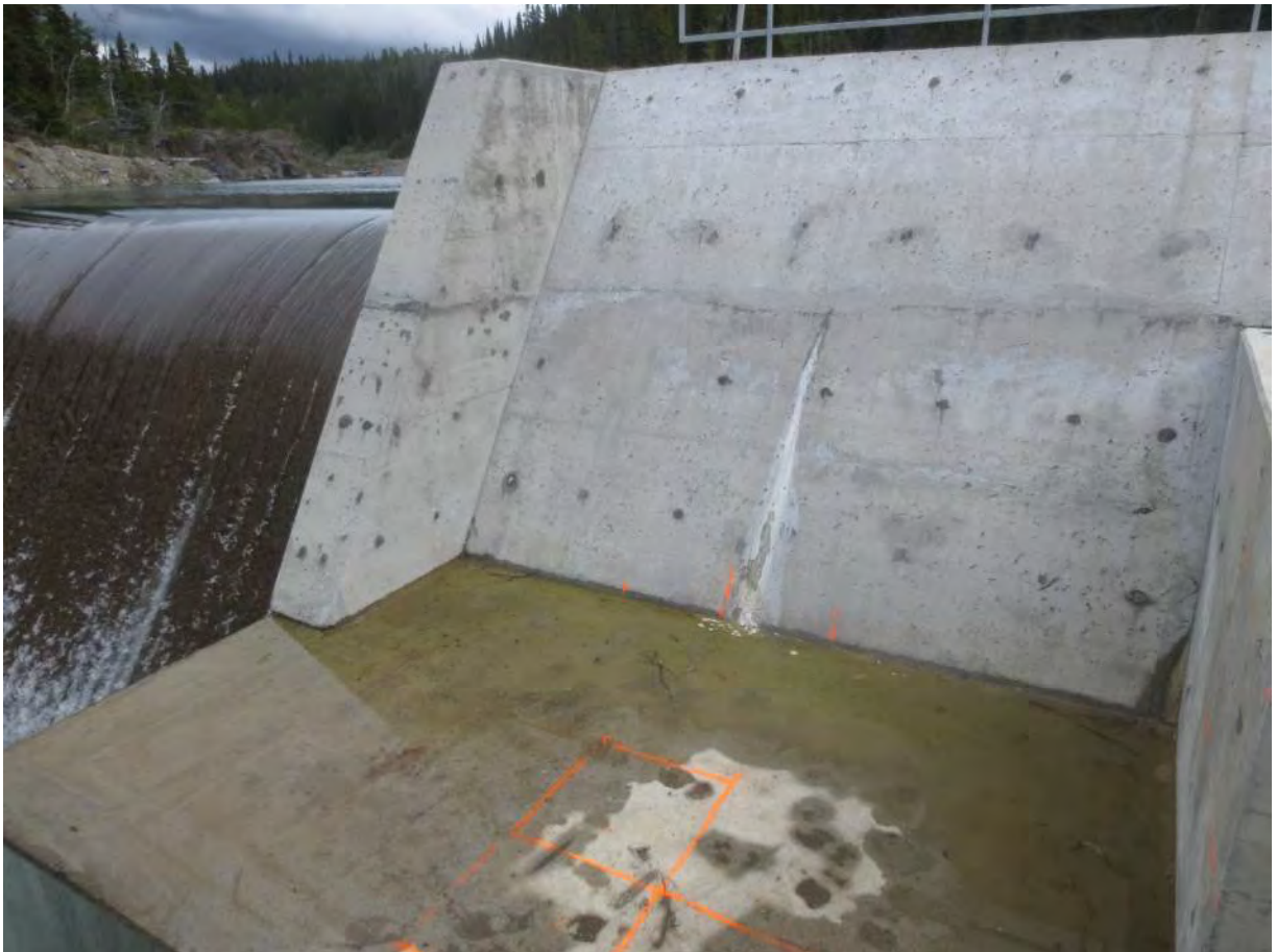
Photo 10: South side of weir. Note minor seepage and efflorescence.
