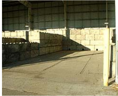
ECS Aeration Floor Port Angeles, WA
