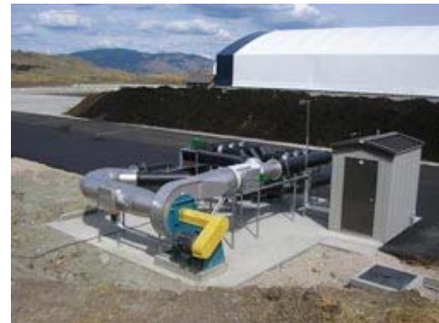
Kelowna Biosolids Composting Facility; Single fan group supplies aeration to six temperature-controlled zones.
