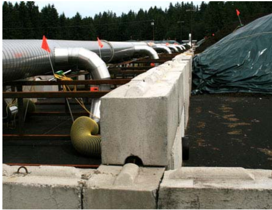
AC Composter™ aeration system with ecology block push-wall
