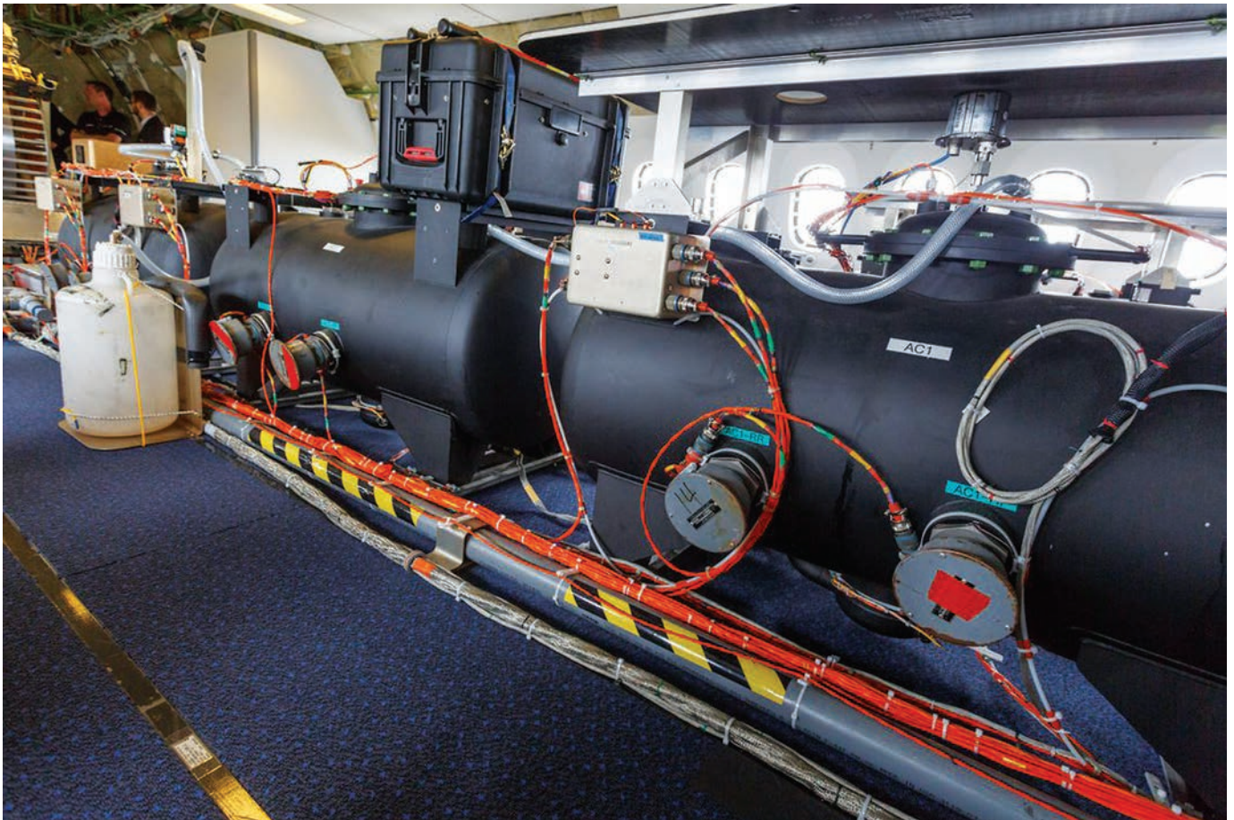
Above: Boeing 787 ballast tanks. Miles of wiring are found on the Dreamliner, but Raytheon's ultimate goal is to reduce not increase weight with the introduction of electrical systems.
