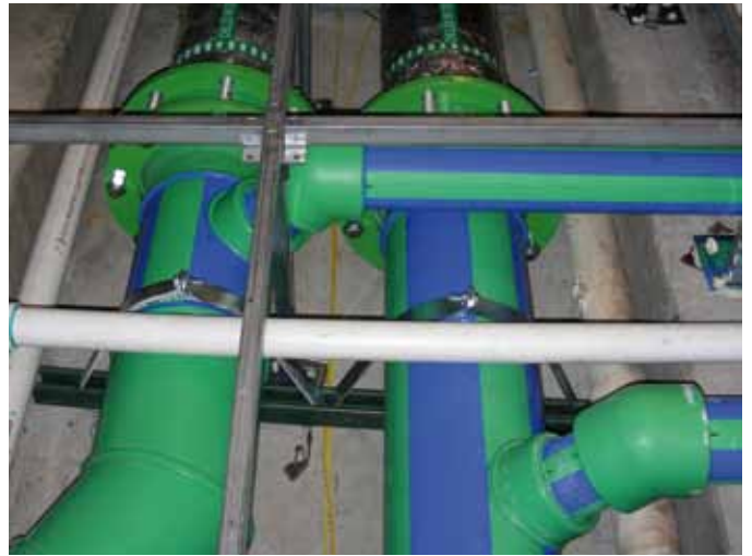
Colorado State University Data Center, USA
