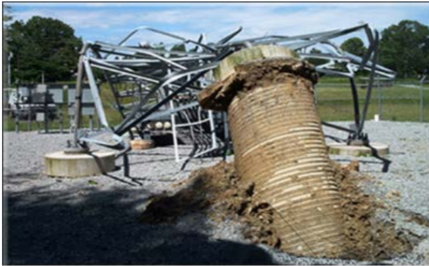
Figure 2.1. Tower foundation failing under effects of uplift and frost
