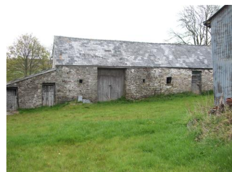
Barn in the Crai Valley, derelict as a result of changing farming practices. Many similar barns throughout the National Park have been converted to residential use.
