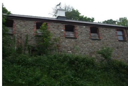
Neglected industrial building alongside former railway line.
