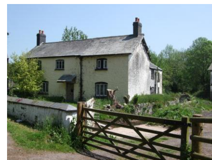
Locally distinctive farmhouse in a poor state of repair
