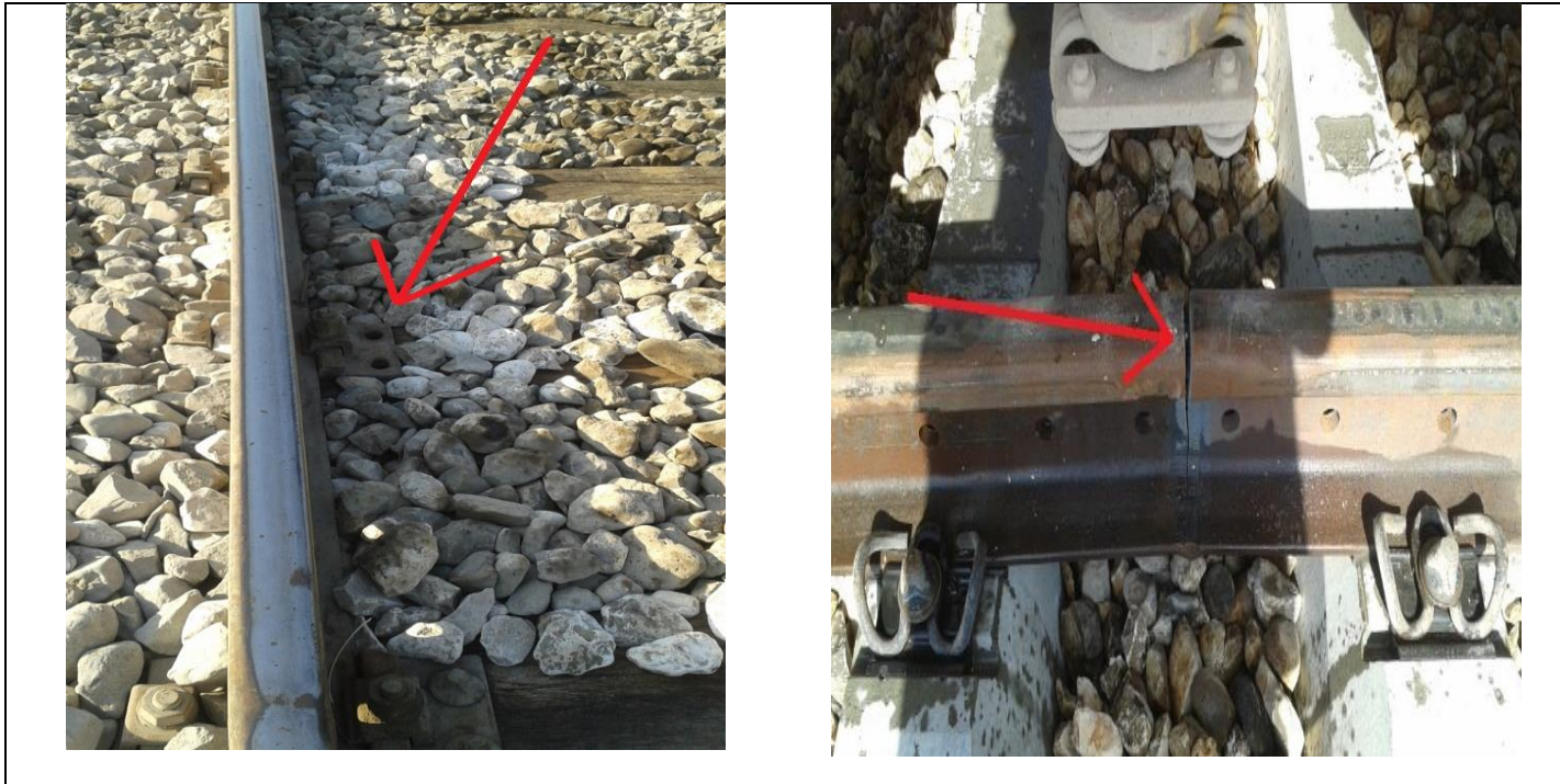
Examples of deteriorated tracks
