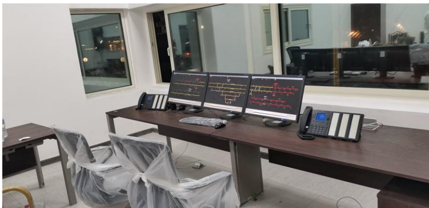
Signaling system after Egypt National Railways Restructuring Project
