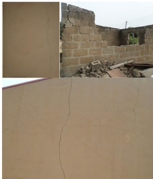
Fig. 9. Samples of the affected structures close to the study area
