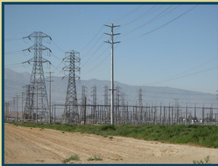
Mira Loma Substation
