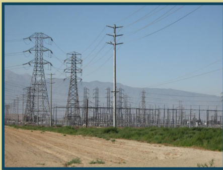
Mira Loma Substation
