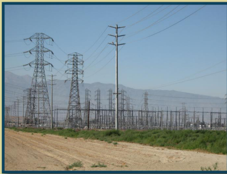
Mira Loma Substation
