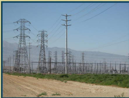
Mira Loma Substation
