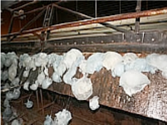
Fig. 27. Jellyfish clogging the cooling system of a power plant
