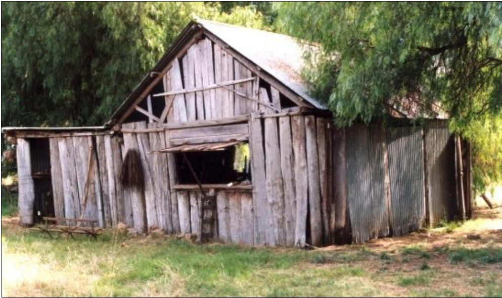
Blacksmith Shop viewed from SE, showing added double doors in the east wall.
