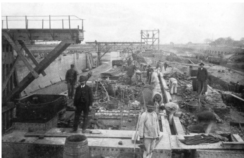
Fig.12. Construction work on the canal locks in Brunsbüttel in May 1893. Photo courtesy of Walter Schulz, Brunsbüttel, Germany (Schulz 1995).
