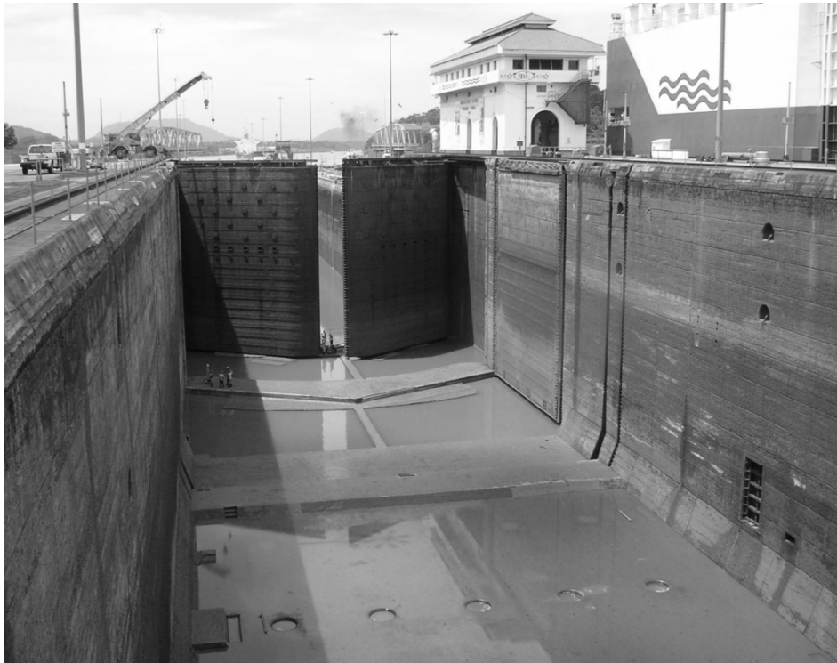
Fig. 3. Miraflores Locks drained for maintenance. The view is toward the lower end of the upper lock chamber. In the center of the image are the two slightly gaping doors of the chamber's lowermost gate: the doors of the gate just above them are folded back into the lock walls. In the foreground are five of the circular wells set into the floor of the chamber through which water enters and drains. Photo courtesy of Mark Torchin.
