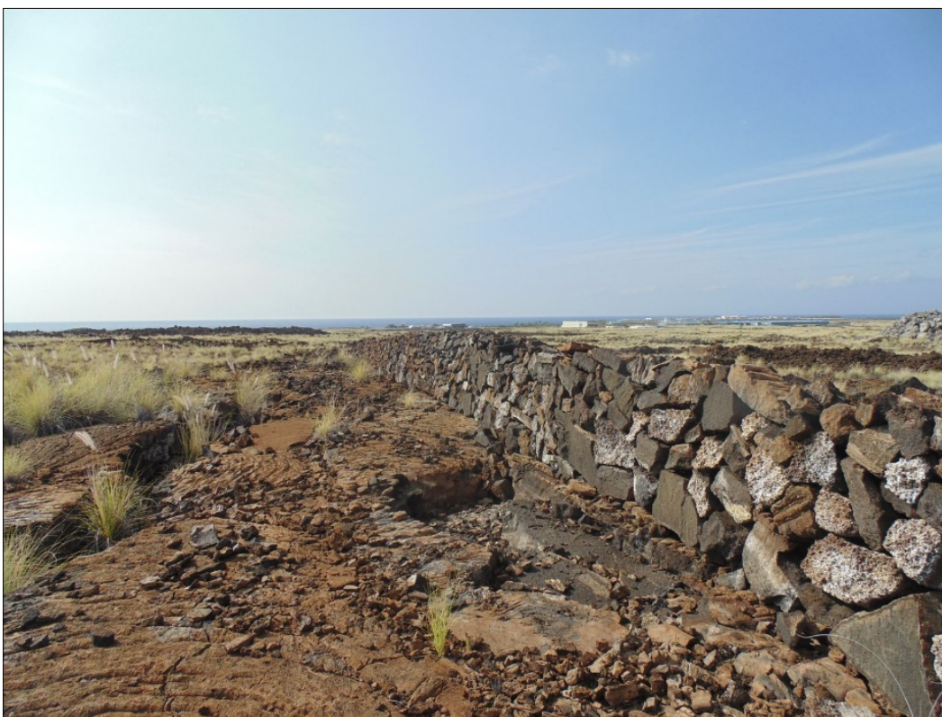
Figure 59. SIHP Site 6432, excavations along the edge of the wall, view to the west.
