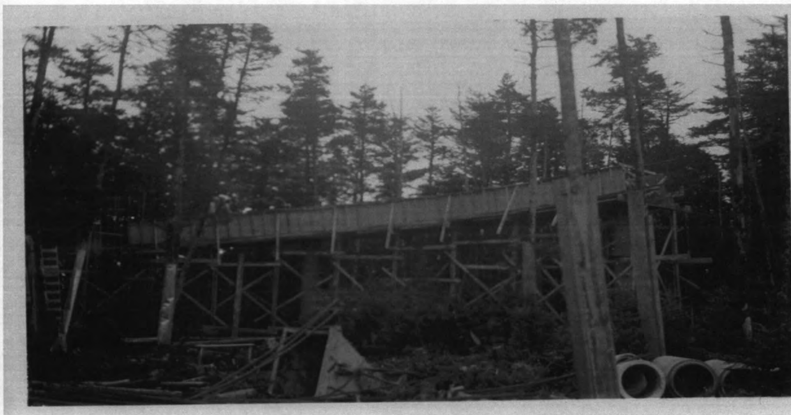
Fig. 6 "Portion of Ramp Showing Forms and Supports" Showing the proximity of trees to the ramp and the protective casings given to several trees. NPS photograph by R.A. Wilhelm, 1959. Archives of GRSM.
