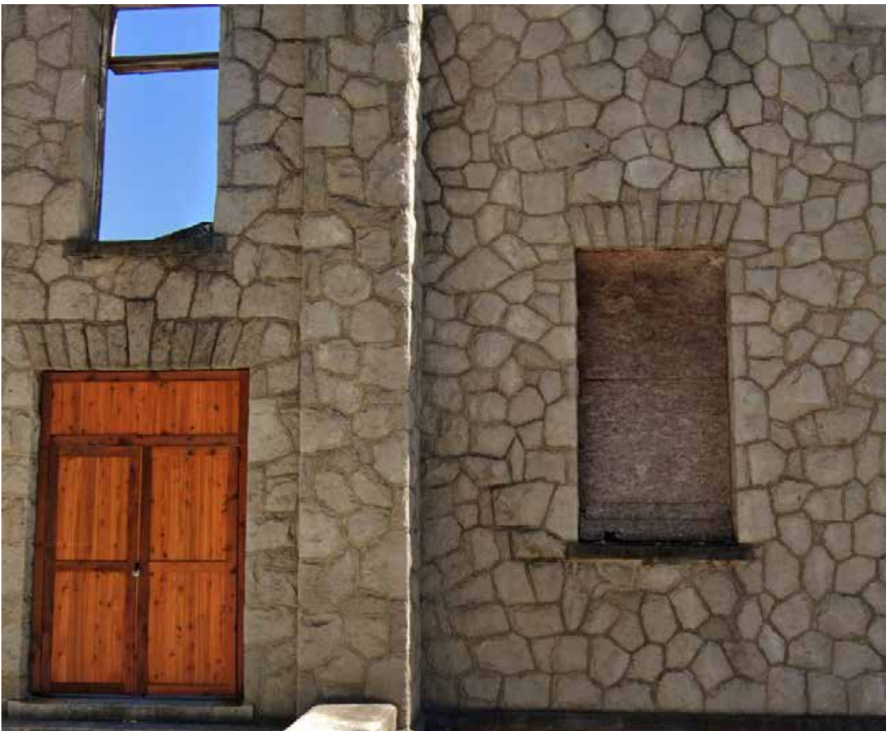
Figure 4.11. Example of similar wall construction at the ruins of First St. Mark A.M.E. Church, located in the English Avenue neighborhood, just north of Vine City. North elevation and closeup of stonework. (Source: Google, 2020.)
