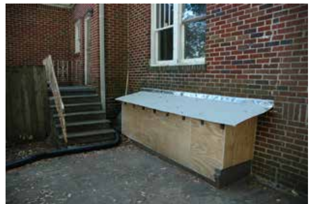
Figure 3.50. Window was enclosed with plywood and flashing between June and October 2019 to reduce the amount of water ingress to the basement and the window well area. View facing east. (Source: HPTC October 2019.)
