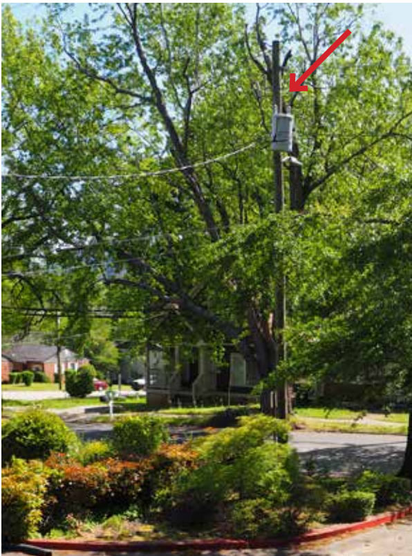
Figure 3.52. View facing northeast of the power pole and overhead residential electrical service in the northeast corner of the site. (Source: WLA Studio, June 2020.)
