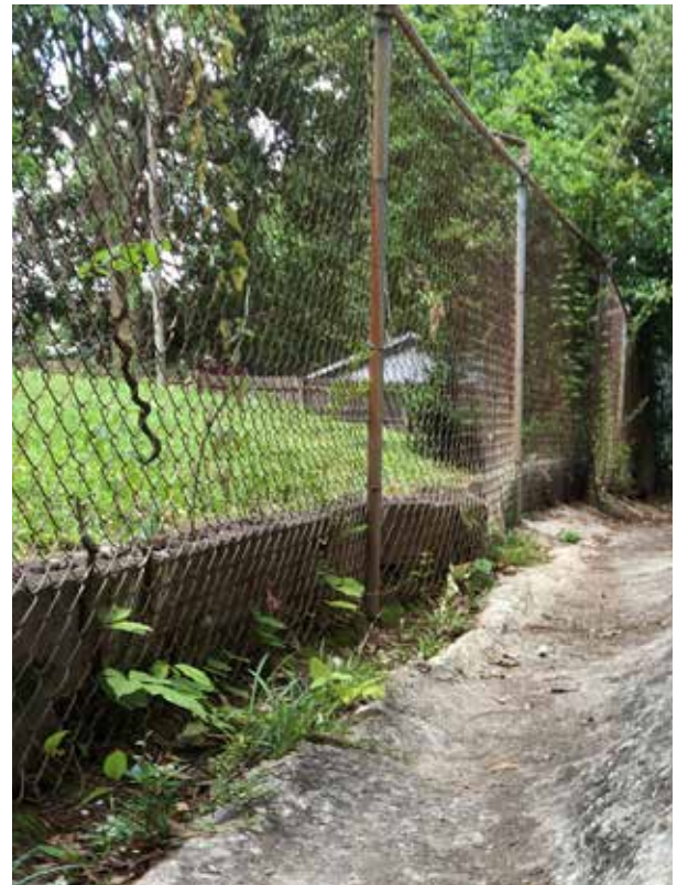
Figure 3.48. Concrete apron/swale on the south side of the house, facing west. Concrete block wall is located south of the swale. Portions of the wall are failing and are being held up by the chain link fence. (Source: WLA Studio June 2020.)
