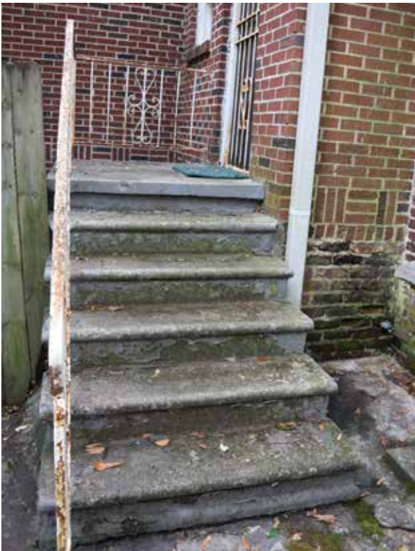
Figure 3.42. View facing east of the brick and concrete staircase located on the north side entrance of the residence. Five concrete risers with a decorative metal handrail lead to a landing. (Source: WLA Studio, October 2020.)
