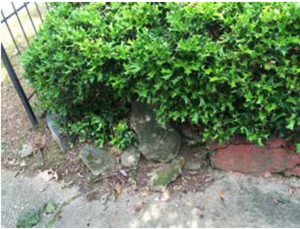
Figure 3.72. Group of stones at terminus of stone retaining wall near southeast property corner. These may be pieces of broken retaining wall. (Source: WLA Studio, April 2020.)
