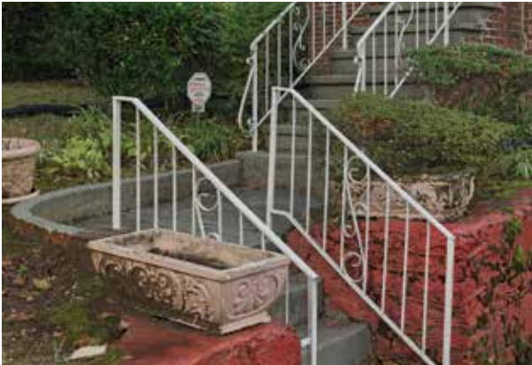
Figure 3.74. Cast concrete planters placed on the stone retaining wall near the steps to the driveway. (Source: HABS GA-199-3.)
