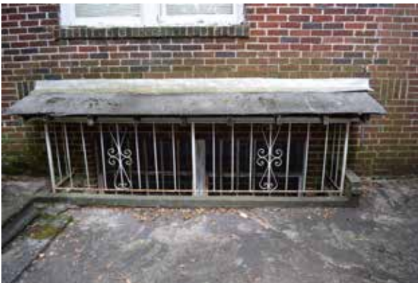
Figure 3.49. A small roofed projection prevents water from entering the garden level window well on the north elevation of the residence. The window well is surrounded by decorative bars that provide security. View facing south. (Source: WLA Studio, June 2019.)
