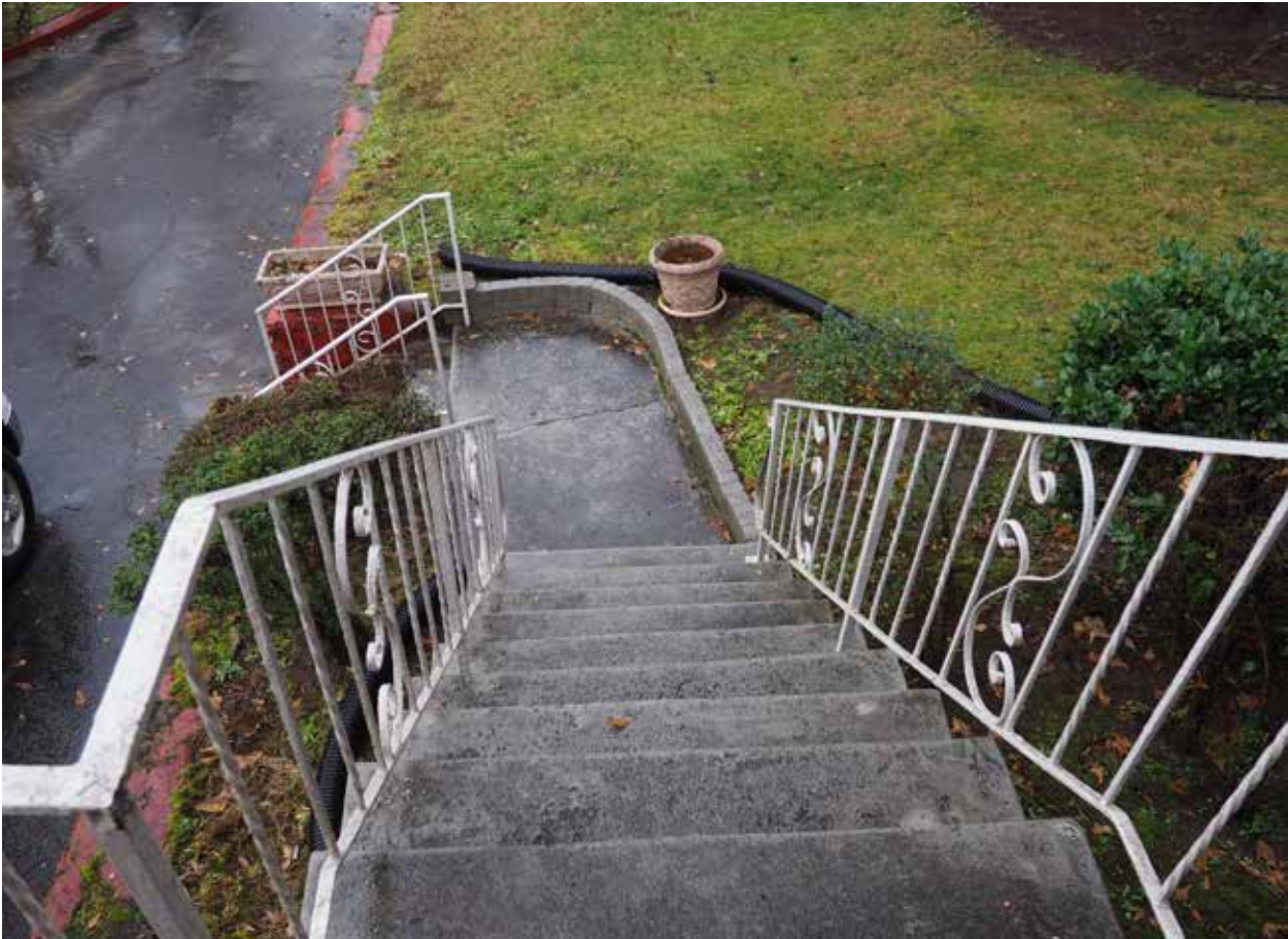
Figure 3.18. View of the curved concrete walkway from the front landing. The walkway is separated from the front turf grass area by a mortared brick edging (Source: WLA Studio, June 2020).
