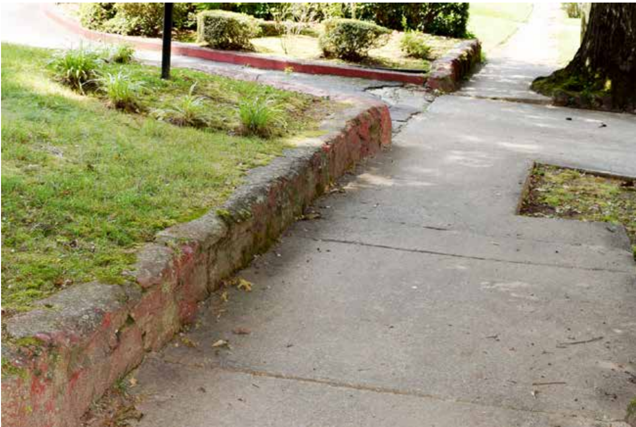
Figure 3.23. View facing north of the stone retaining wall, which holds the grade between front turf grass area and sidewalk. The stone wall turns ninety degrees at the eastern edge of the driveway. The wall is present on both the north and south sides of the driveway. The concrete sidewalk is six feet wide in most areas. (Source: WLA Studio, June 2019.)
