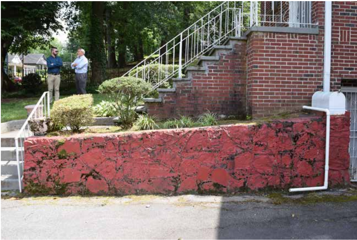
Figure 3.45. Western portion of the stone retaining wall, which lines the south side of the driveway. View facing south. (Source: WLA Studio, June 2019.)
