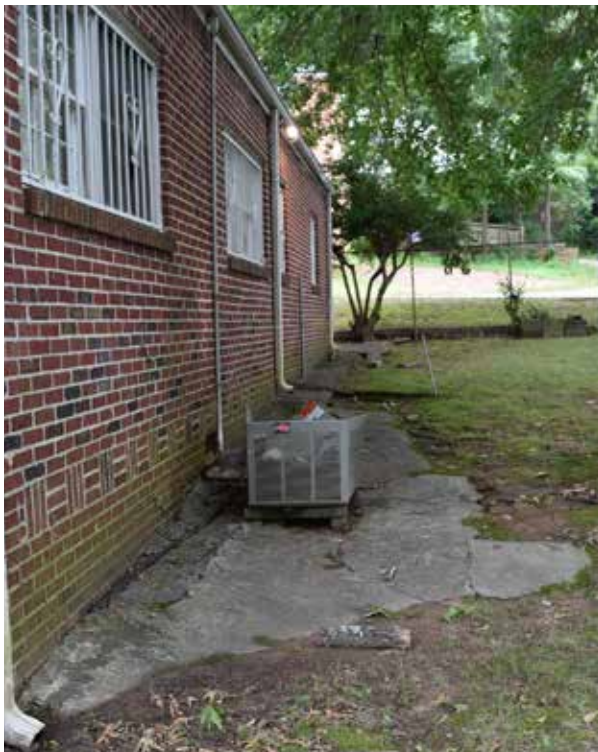
Figure 3.66. Concrete apron on west side of the house (rear yard), facing south. (Source: WLA Studio, June 2019.)
