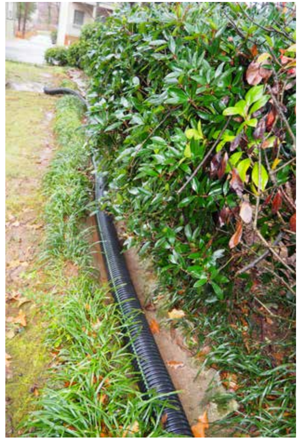
Figure 3.69. View of the concrete swale in the front yard, which now contains a temporary drainage pipe. (Source: WLA Studio, April 2020.)
