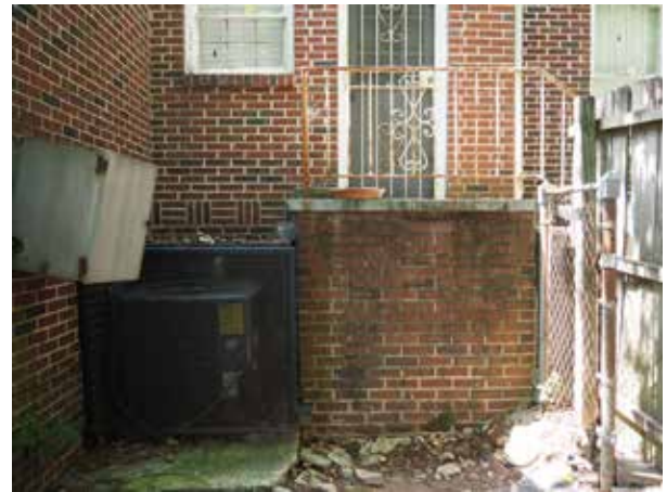
Figure 3.53. HVAC Unit located inside cage structure on north elevation. (Source: WLA Studio June 2020.)
