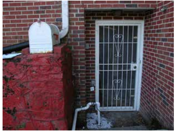
Figure 3.73. View of the sump pump and mailbox at the basement entry door. The sump pump alleviates moisture at the basement level of the house. (Source: HPTC, October 2019.)
