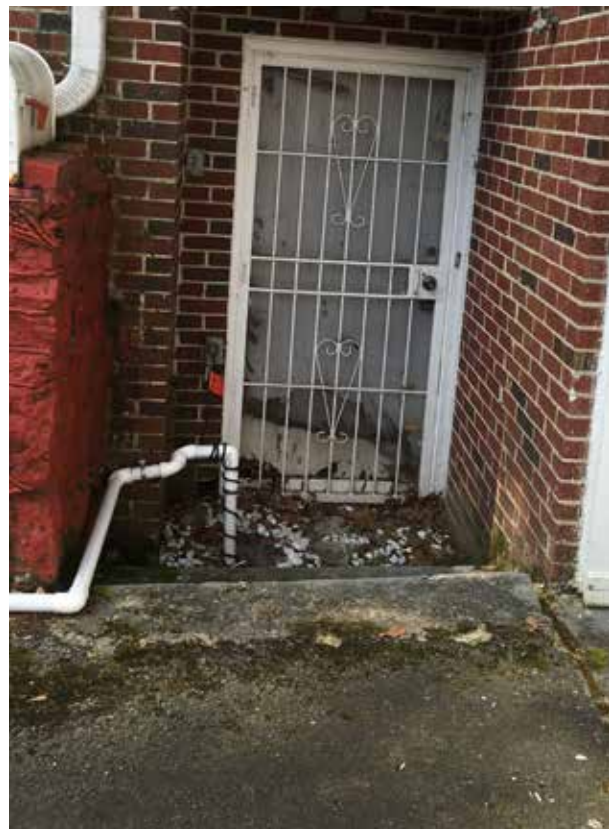
Figure 3.16. Concrete step leading to basement entry door, facing south. (Source: WLA Studio, June 2020.)
