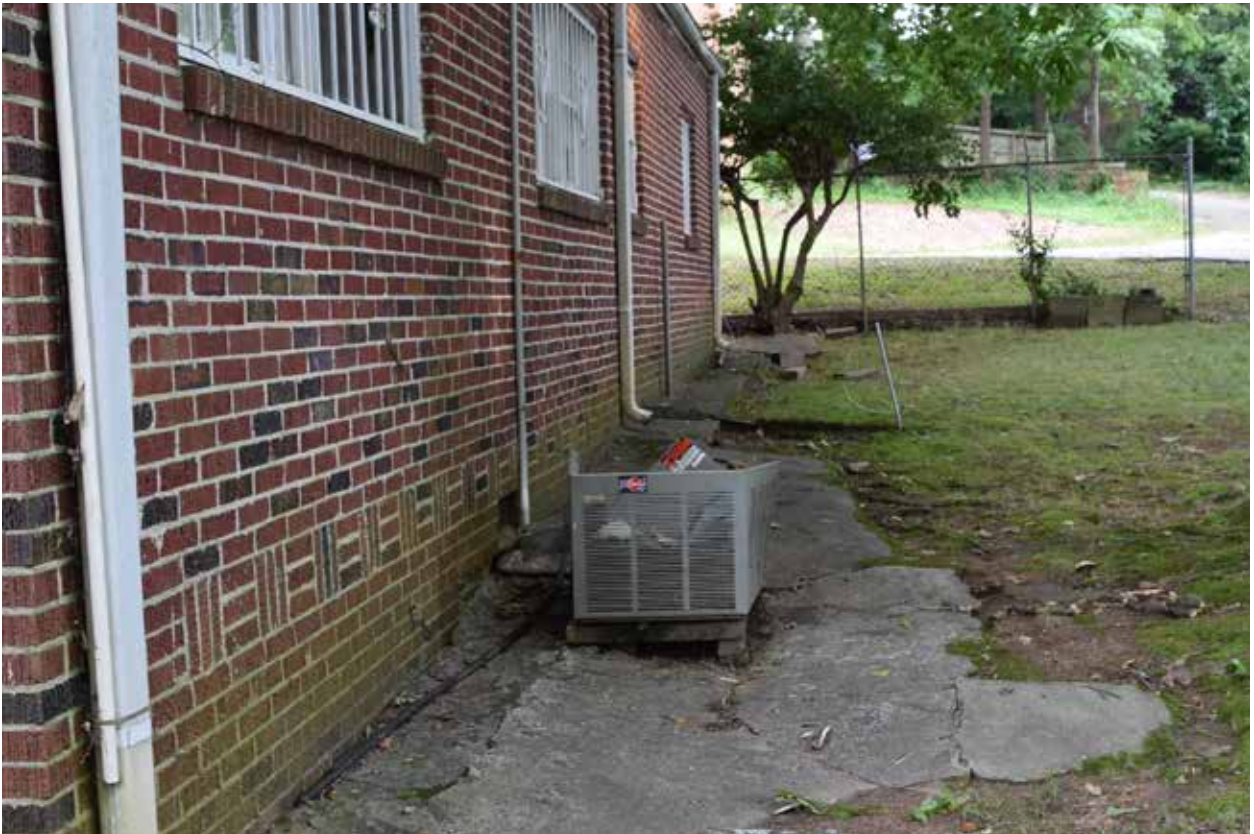
Figure 3.54. Nonfunctioning HVAC unit located in rear yard, facing south. (Source WLA Studio June 2020.)
