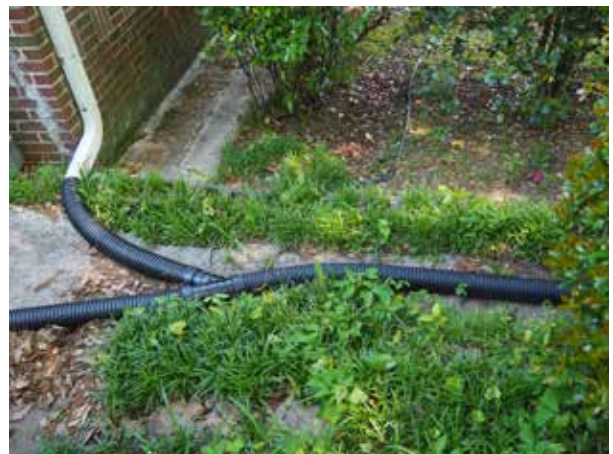
Figure 3.77. Because concrete apron and swale no longer direct water away from the house foundation, the NPS has added drain pipes to direct water toward Sunset Avenue. (Source: WLA Studio, June 2020.)
