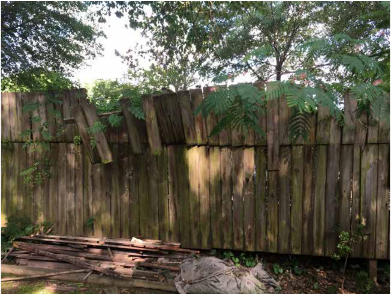
Figure 3.61. Wood privacy fence in the back yard has been modified, likely for privacy or security, on the western boundary of the property, facing west. (Source: WLA Studio, June 2019.)
