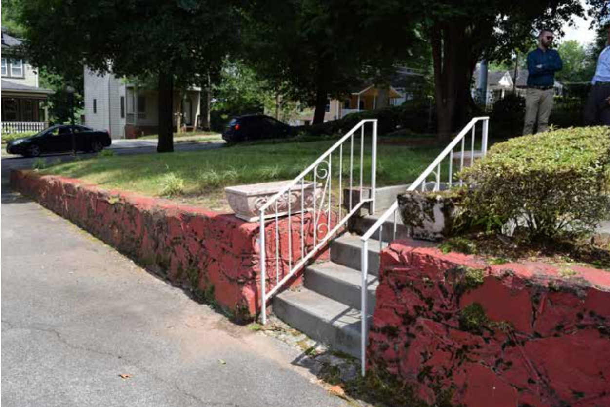
Figure 3.46. View of retaining wall, facing southeast toward Sunset Avenue. (Source: WLA Studio, June 2019.)
