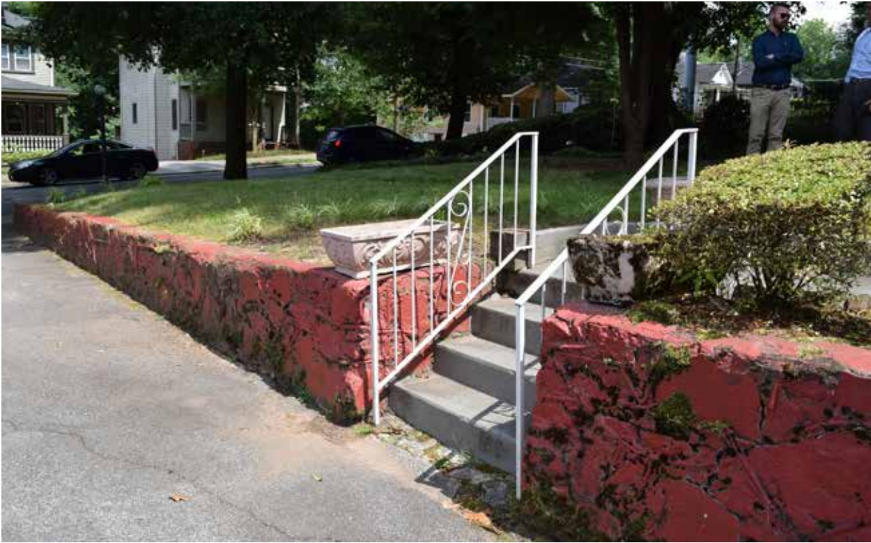
Figure 3.22. View facing southeast of the stone retaining wall, which holds the grade between front turf grass area and driveway. The wall terminates into the grade on either side of the staircase. (Source: WLA Studio, June 2020.)
