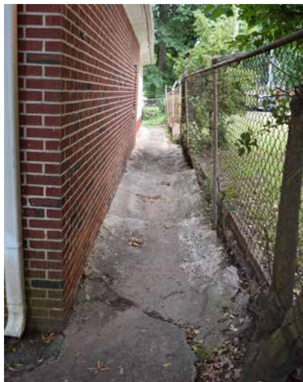
Figure 3.67. View of the concrete apron on south side of the house, facing east. (Source: WLA Studio June 2019.)
