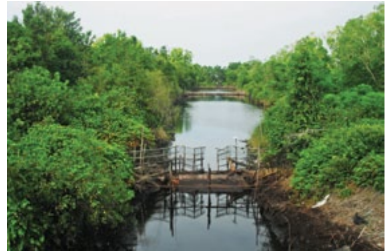
FIGURE I 5 Successive ditch blocks made of wood and soil bags in a medium-width canal in Central Kalimantan.
