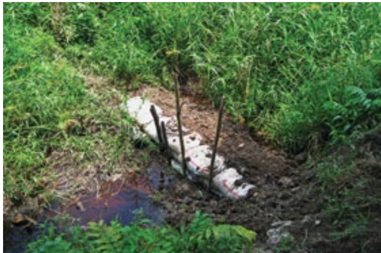
FIGURE I 4 Small ditch blocked with sandbags and soil.
