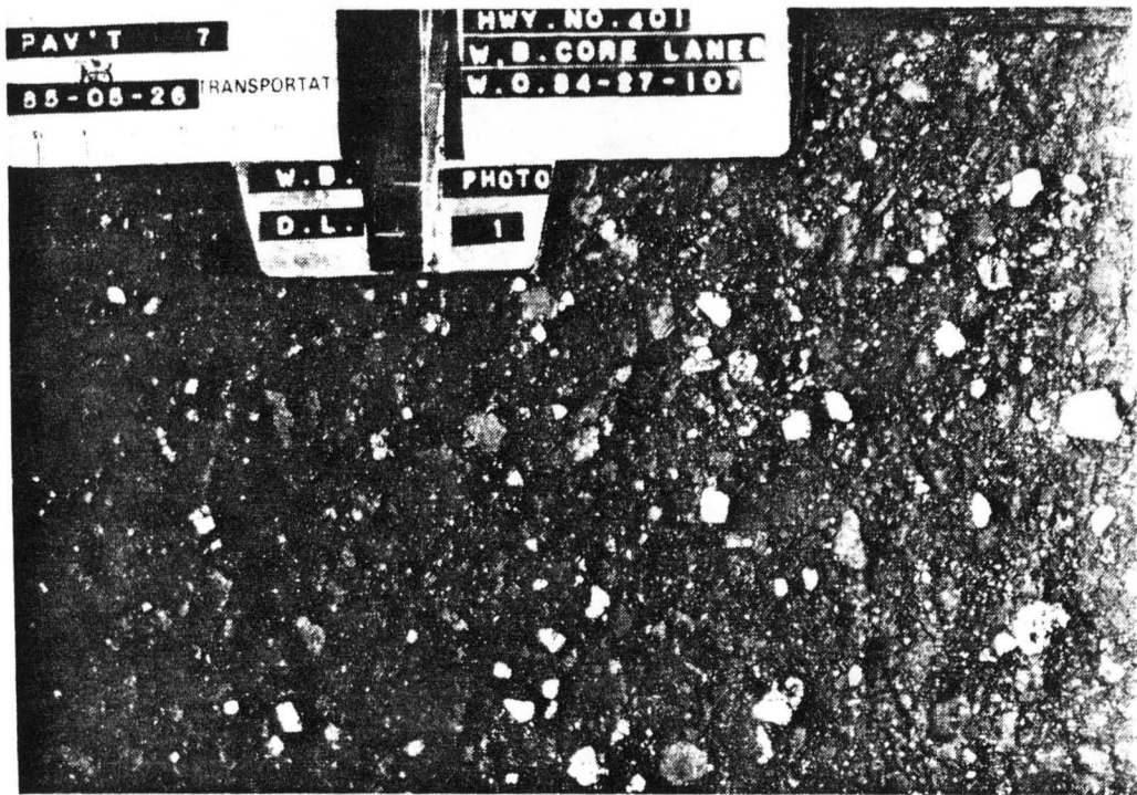
Fig. 4: Close-up of Test Section No. 7, Wheel Path, Driving Lane, After 11 Years Service Friction Excellent, Good Macrotexture and Microtexture Steel Slag Coarse Aggregate Steel Slag Screenings Fine Aggregate
