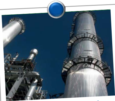
Energy Verbund >€300 million annual cost savings
