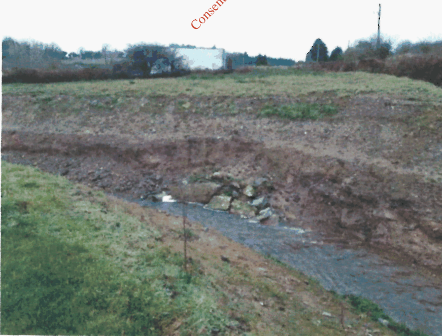
Figure 1. Collapse of bank slope
