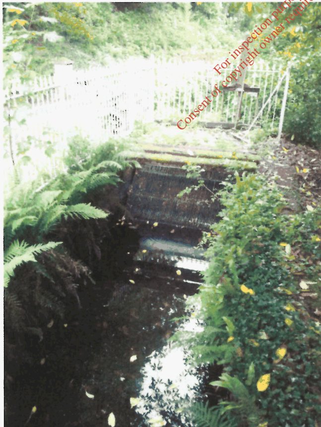
Photo 8. Screen and sluice on the lake outflow channel.
