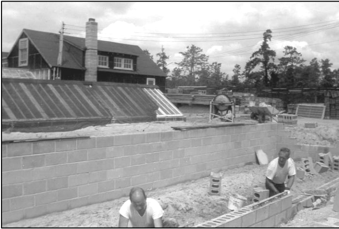
Jack Cadbury III (front) and Mark Cutts (back) laying block for the second greenhouse at Holly Haven Inc. The lath house is on the right and the sash house complex is on the left, June 1955.
