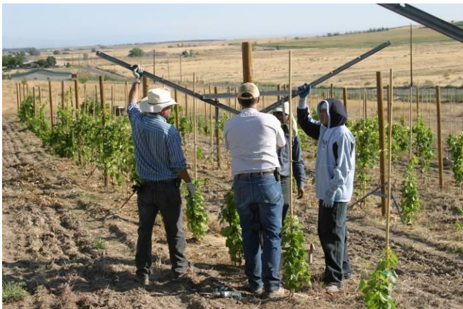
Photo 46. Installation of an Arbor or Slanted One-sided cordon arms system at the University of Idaho. Cordon wires at about 57 Inches above the ground.
