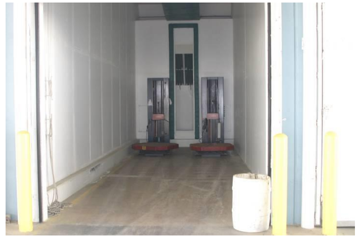
Photo 151. SO 2 gas room for disinfection.
