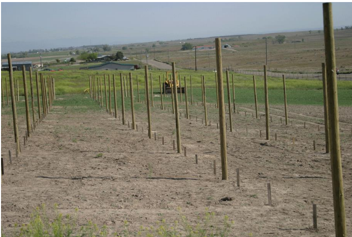
Photo 21. Support posts (in posts) are installed and places for vines are marked before planting. This is a preferred method in Idaho.
