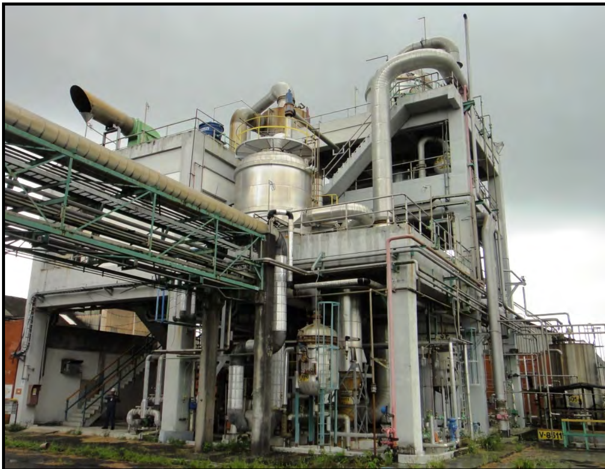
Ammonium Sulfate Plant
