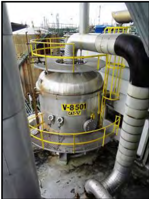
1st Stage Evaporator
