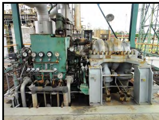
Process Air Compressor
