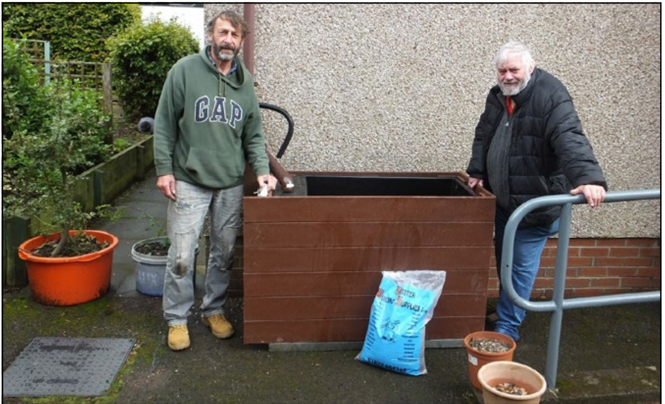
Local Mr Fix-it Julian Foster, and design engineer Neil Campbell, installing the raised bed rain garden.
