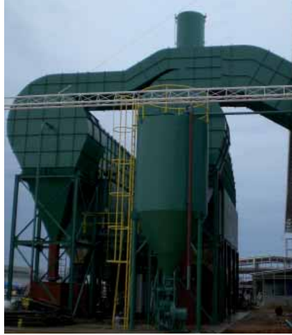
Alva Aluminium, Tailandia FS722 / 9,00 / 1260 with Skimmer, Lime feeding and recirculation system, for 2 gas fired tilt rotary furnace
