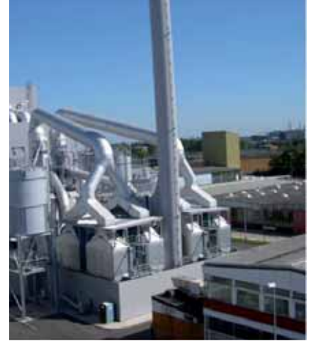
Harpen EKT, Berlino (Germania) Wood fired power plant "Gropiusstadt" Emission Data: dust < 5mg/m 3
