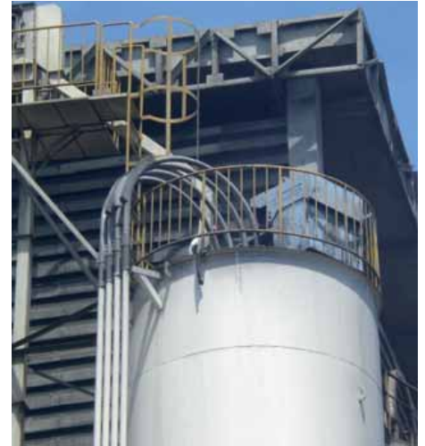
SiloSafe on Silo SiloSafe on fly ash silo
