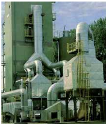
FLS, Germania FS Filter for temp 135 deg. C Application: fume gas cleaning for garbage incineration
