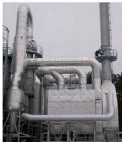
Otto-Rudiger Schulze, Wilmersdorf (Germania) Biomass power plant, air volume max. 58,000 Nm 3 /h Temp. boiler end 180-200°C, SO x , HCl in raw gas
