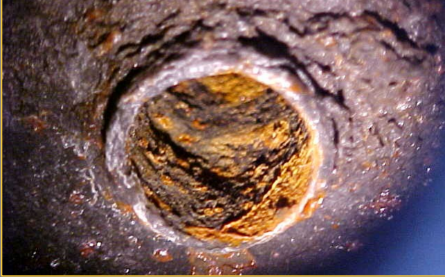
Heavy fouling and tube end corrosion
