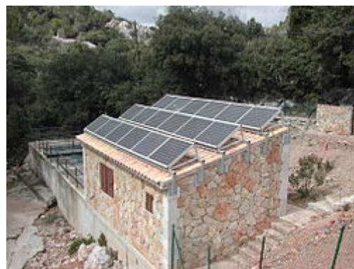
A sewage treatment plant that uses solar energy , located at Santuari de Lluc monastery, Majorca
