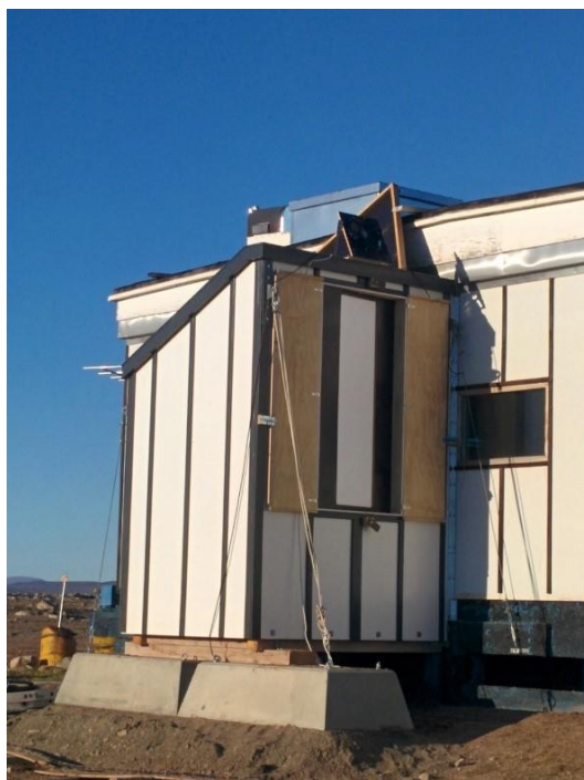
Figure 3.9: A photo of the exterior of the wooden annex hosting VESPA-22. The observing window of the signal beam is visible on the side of the annex. The fan blowing on the zenith windows can be seen on the roof; the other fan was not yet installed at the time this photo was taken.
