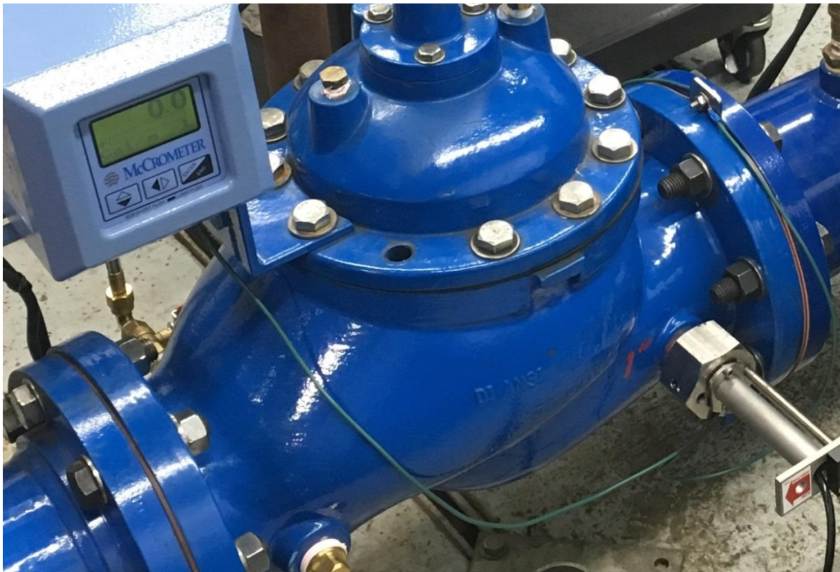
Figure 26: Converter & probe with ground wiring
