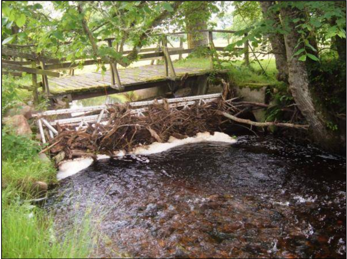
Plate 5 Water gate trapping debris on Belladrum. Such obstacles can prevent upstream migration by adult fish and represent potential sources of mortality to smolts etc migrating downstream.
