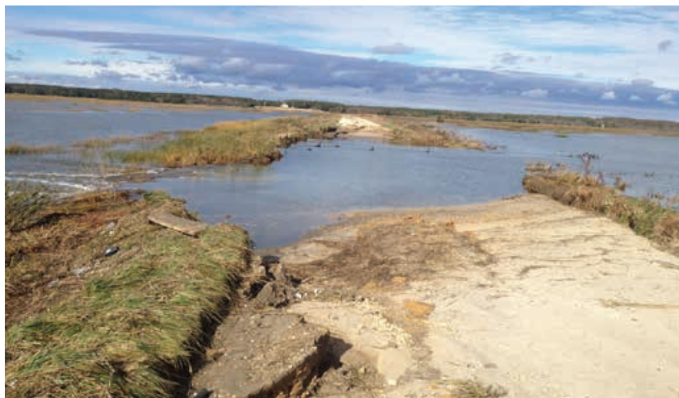
Talk about disturbance. Hurricane Sandy's eye went directly over Wildlife Drive at Edwin B. Forsythe National Wildlife Refuge in New Jersey and left this damage to the eight-mile auto tour loop. (USFWS)
