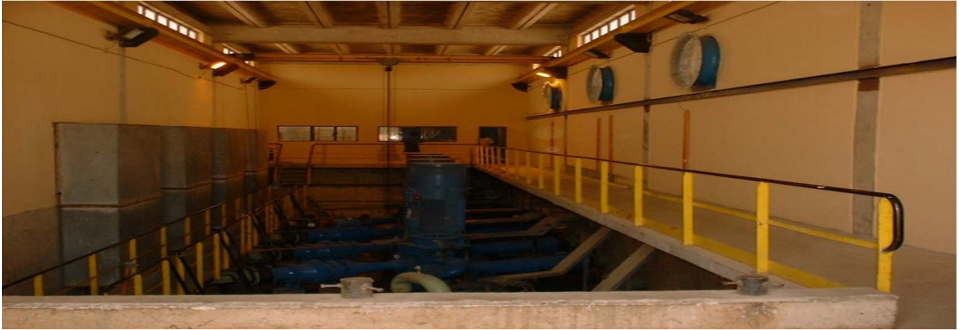
Bauchi High lift Township Water supply pumps
